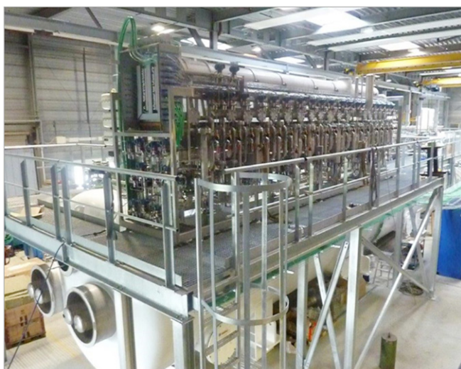
Figure B.4 CTCB at factory for mechanical factory acceptance test (FAT)
